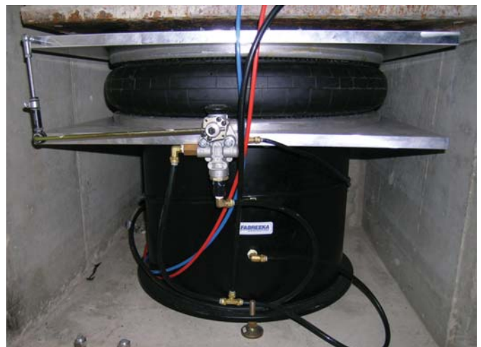
Single convolution air bag isolator with damping chamber and leveling valve supporting a reaction mass for electrodynamic shaker.
