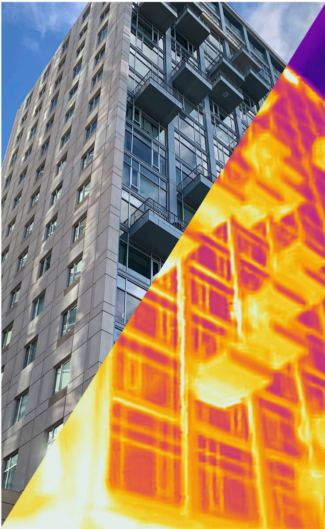
Pictured here: A side-by-side comparison of a building envelope and the heat map throughout the structure without the use of thermal breaks.
